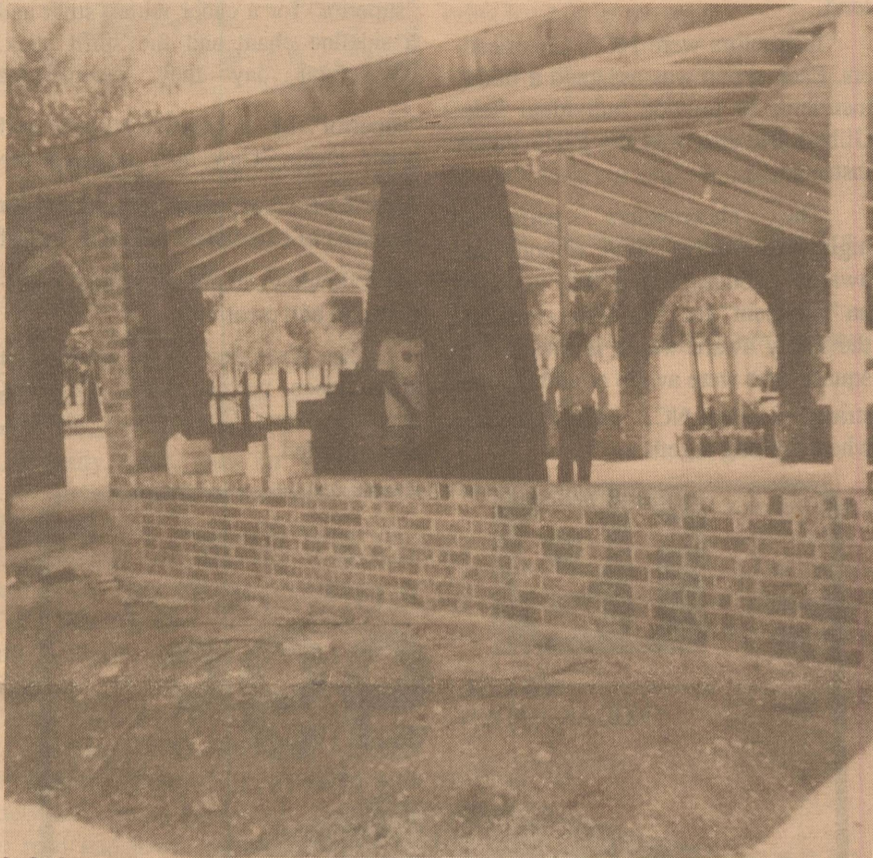
GAZEBO GOING UP - Construction continues in Stanford Park for a gazebo donated by First Christian Church. The gazebo will be dedicated during the Old Settlers' Reunion Saturday, Aug. 3.
