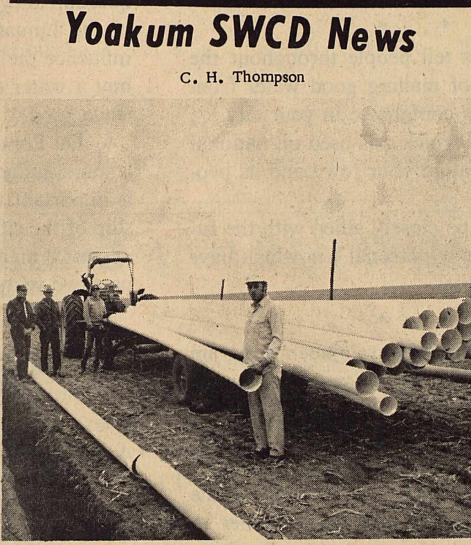
Installing underground irrigation pipeline on the Yoakum Farm Company land in SW Yoakum SWCD. John Milligan of Yoakum Farms and Gilbert Pierce of The Plains SCS with two laborers are shown with part of the pipe being laid. SCS Photo
