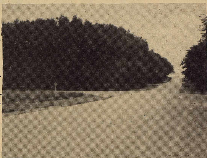
Retopping that has been done on the road west of Stanford Park.
