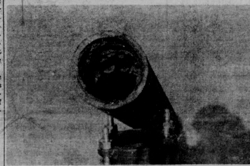
BELOW: This is the reason the mains need cleaning. This section of six inch pipe is almost closed by the development of "tubercules" of rust and mineral deposits.
