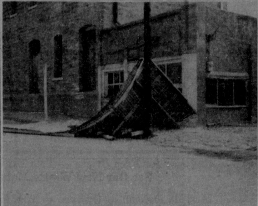
WIND DAMAGE resulting from a thunderstorm front that struck Santa Anna Friday afternoon, along with more than an inch of rain, was scattered. Above, the awning over a cafe in the 100 block of North Second Street collapsed under the buffeting of the wind.
