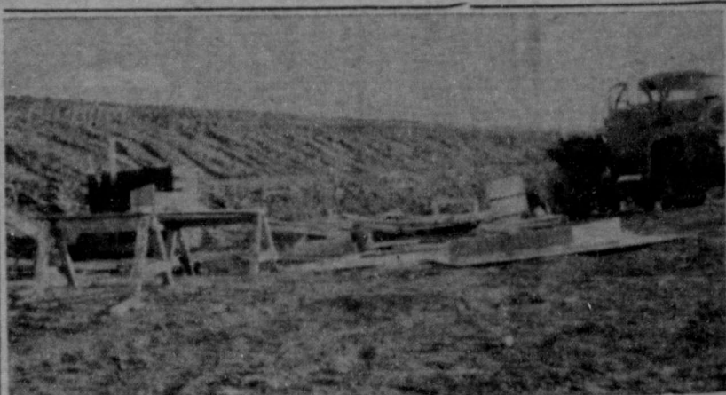
UNDER CONSTRUCTION, this will be a small watershed structure on the property of Mrs. Kate McIlvain, near Rockwood. The structure will assist in flood control, will conserve water by preventing wasteful runoff, and will provide recreational potential. This is one of 22 such structures on the Home Creek Watershed.
