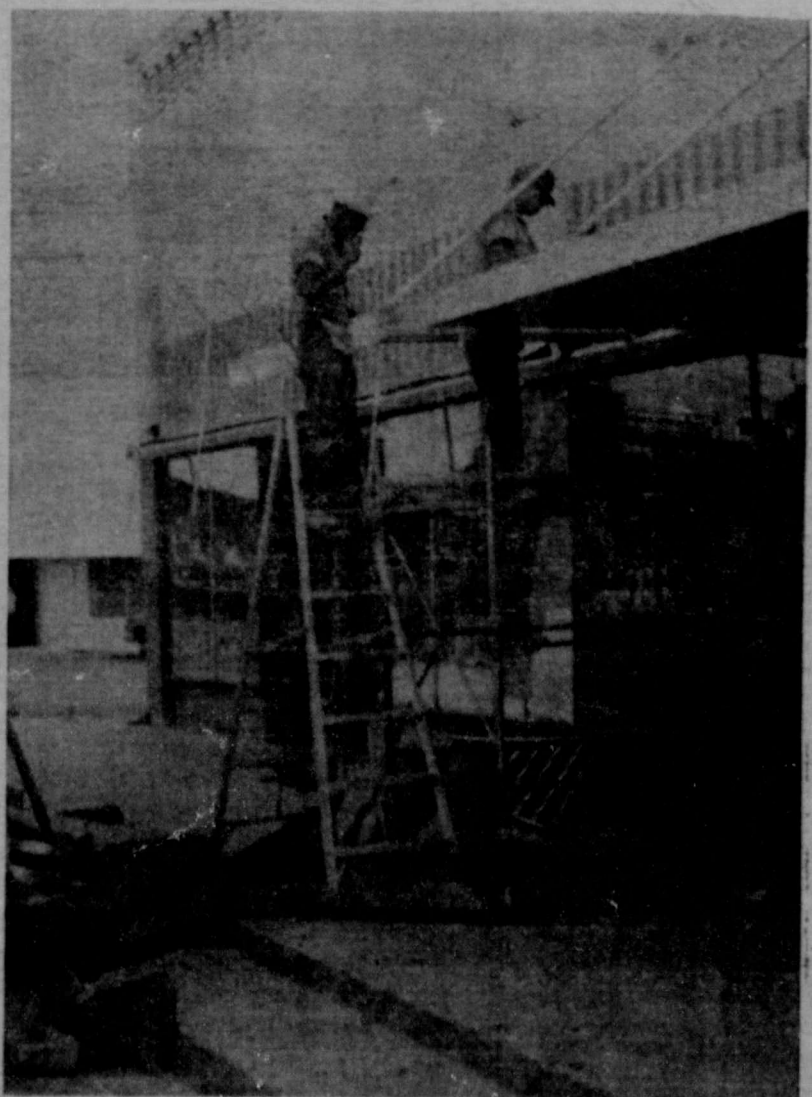
FACELIFTING going on at Hosh Grocery and Hosh Furniture Store is pictured here. Included in the plans are a new awning, new window facings, new metal and glass doors, and a general beautifying of the front of the two stores. Located on the corner of Wallis Avenue and 1st Street, the new facades will add considerably to the appearance of downtown Santa Anna.
