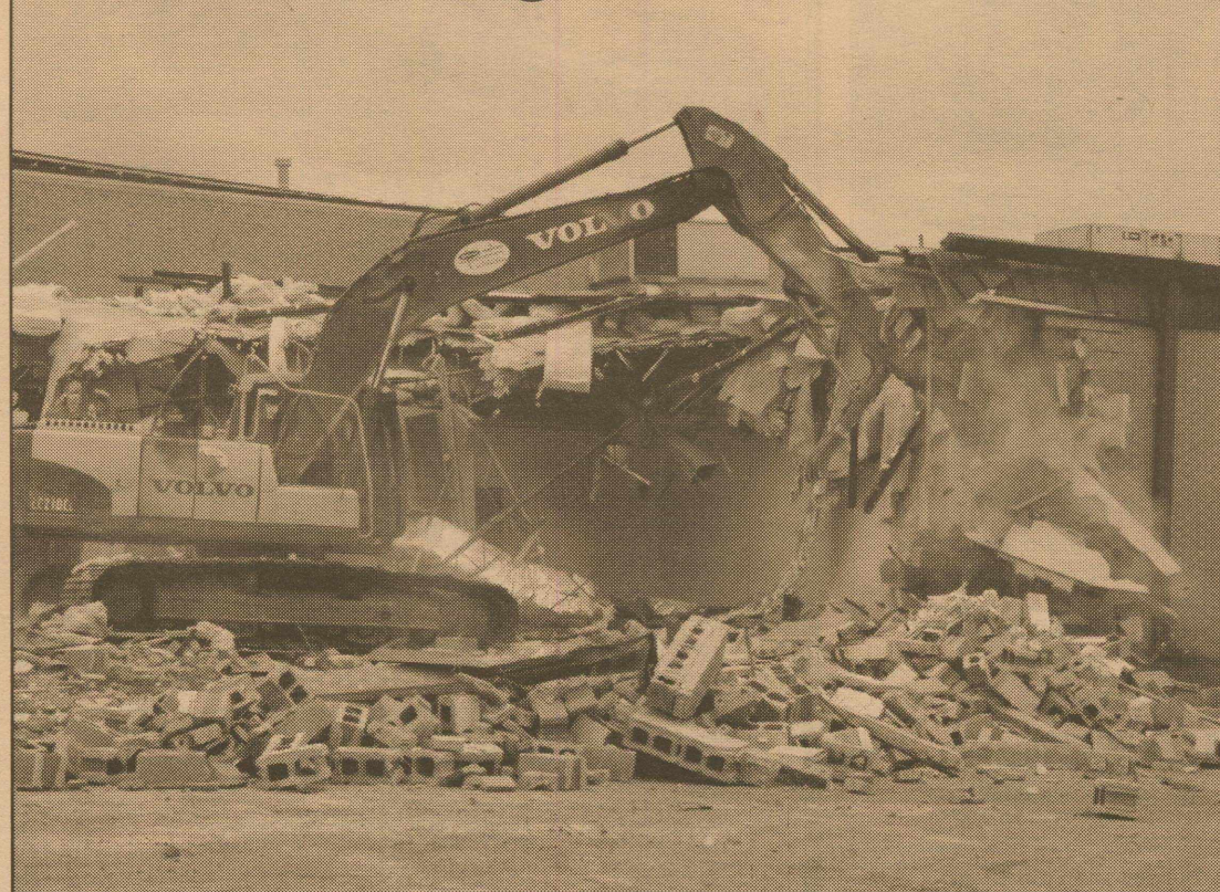
Crews are pictured knocking away the outer wall of the Home Economics department as they began the demolition of the old school building this week.
