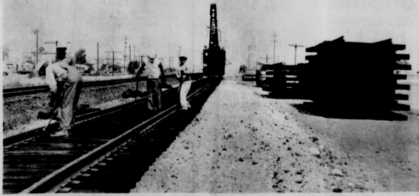
LAYING TRACK—It has been since the 1880's that railroad track has been laid in this county, with the exception of repairs made after derailments, but pictured above is a scene of modern day track being laid. Section Foreman H. P. Lockeby of Clarendon is overseeing the laying of 1.3 miles of passing track in northwest Memphis. The 33-foot track and ties sections are stacked on the right of the picture. The Crane positions them and crews fasten them together. Mr. Lockeby's five-man crew is from Clarendon. Also assisting is a 5-man bridge crew which has been stationed here to rebuild a bridge just south of Memphis. Ft. Worth and Denver R. R. will be shipping coal trains soon on the track and the passing track will be put to a lot of use.
