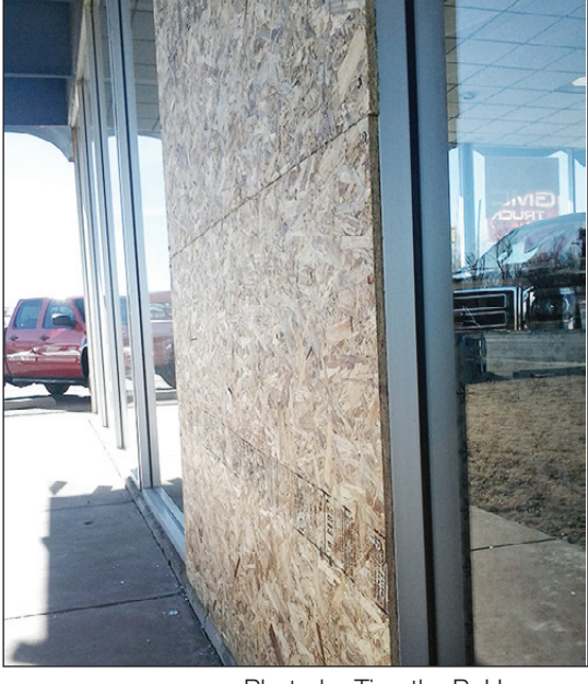
Photo by Timothy P. Howsare Plywood temporarily covers the shot out showroom window at Culberson-Stowers.
