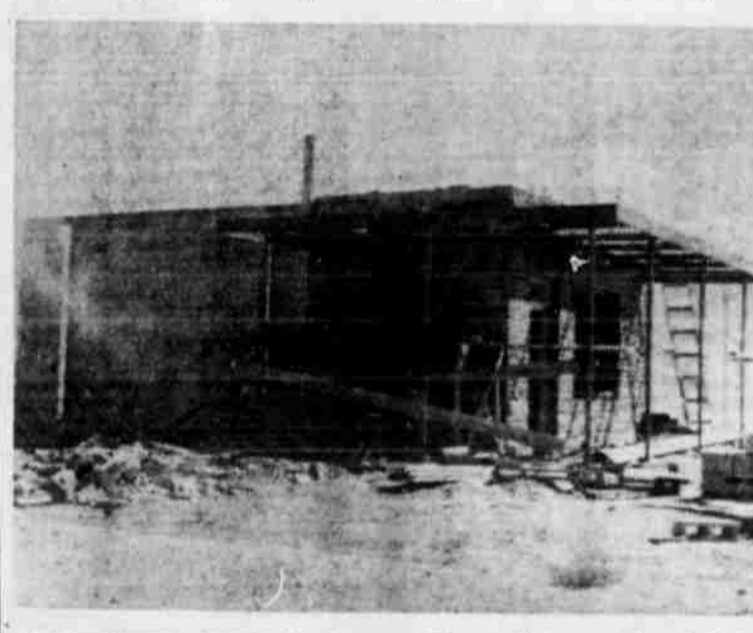
PRESENTED HERE is the new Faust clinic and hospital is being built at Earth by Dr. and Mrs. F. B. Faust. Dr. Faust is a heart specialist and formerly practiced in Littlefield. The new clinic and hospital is of concrete blocks and steel construction with a front of ornamental stone.
