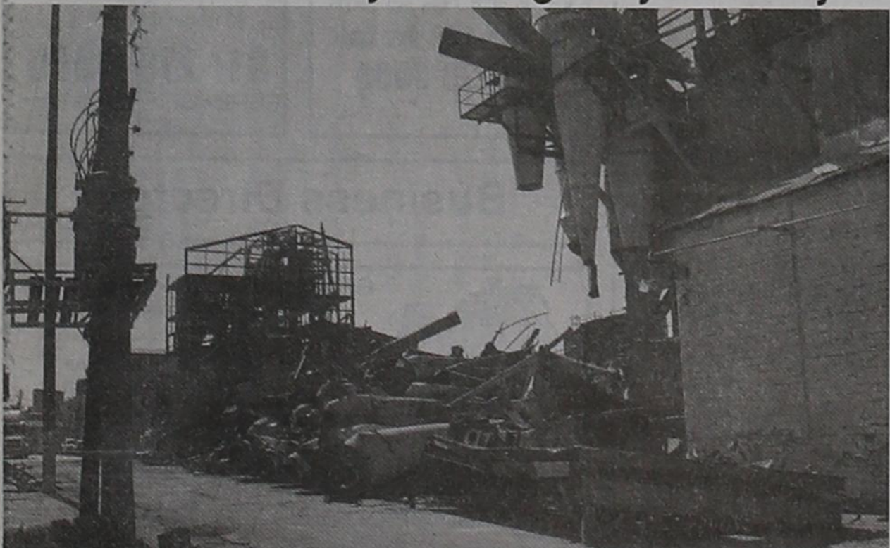
The old buildings for the original Shell Peanut Company and then Birdsong Peanuts are saying goodbye as they are being demolished. The buildings have been a part of the Gorman skyline for a long time. Sad to see them go.
