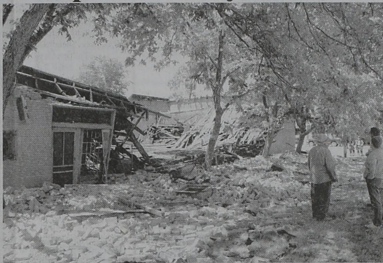
The Blair Building above once held a general store to buy all type of goods in the early 40's and 50's. The Building was being used for mostly storage until the collapse. The front of the building left standing was finally pushed down later.
