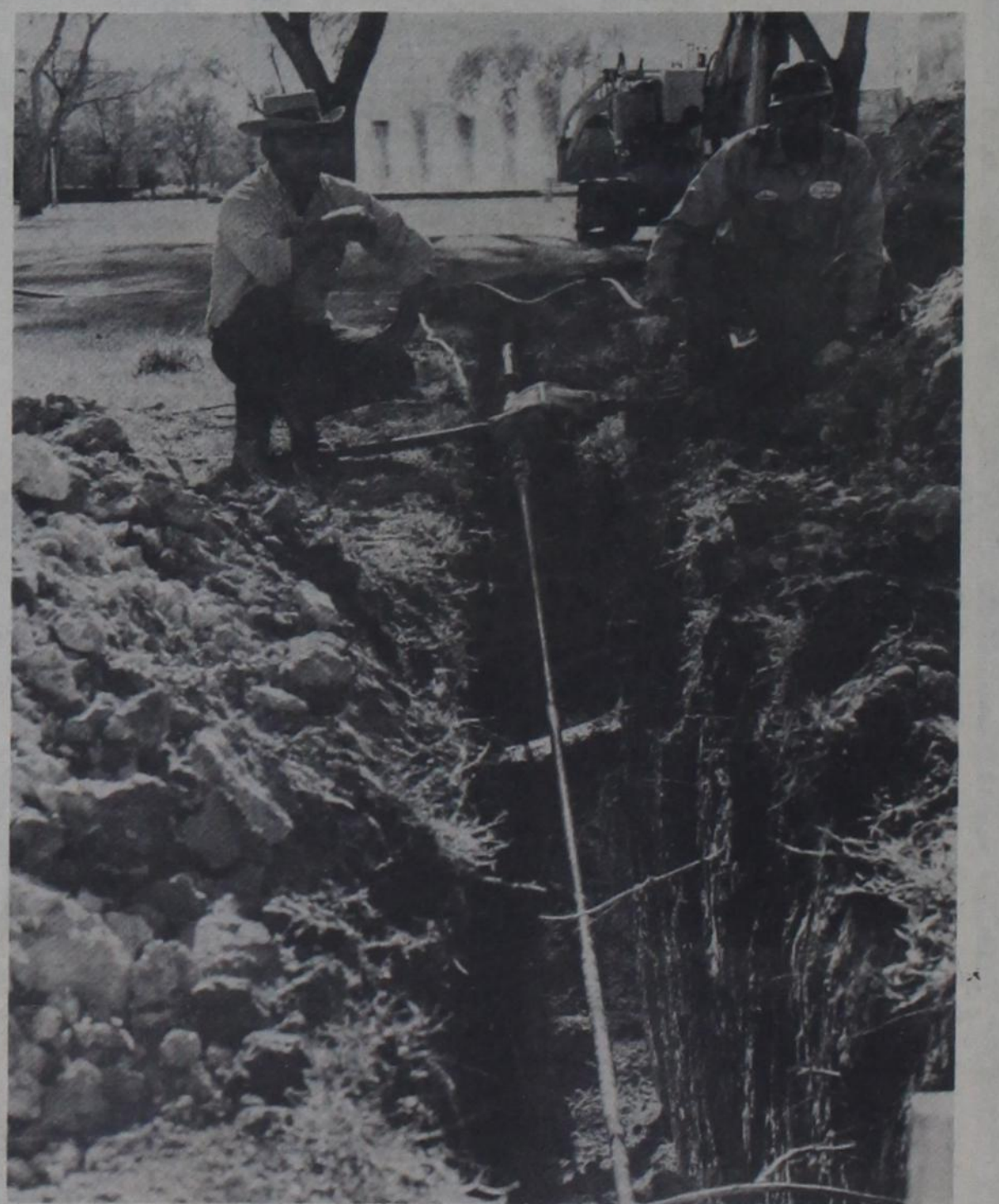
TELEPHONE WORK-If you've wondered about the trenching being done on the east side of campus, it's just Ma Bell burying more cables in an area telephone service expansion. (UD photo by Pat Broyles)
