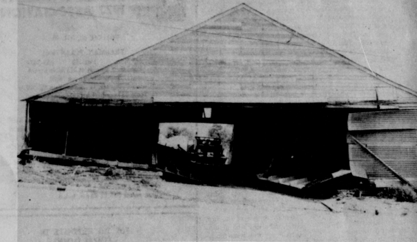
THE PORTER BARN PREPARES TO "BITE THE DUST" AS Baker and Taylor crews prepare to demolish the structure.
