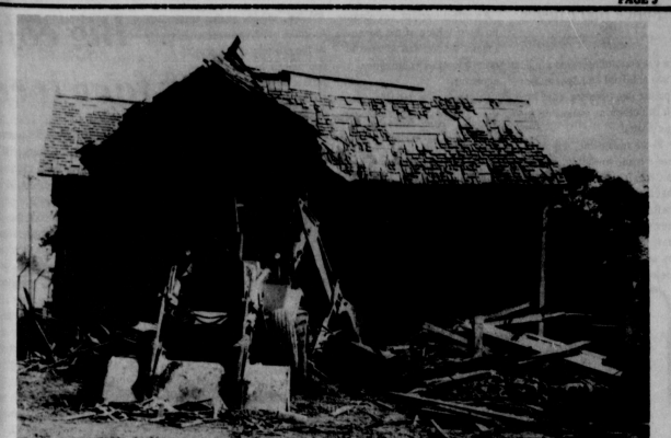
THE FIRST HOUSE ever built in Hansford County, was purchased by Jr. Lusby, and promptly demolished in Spearman's clean-up paint-up campaign.
