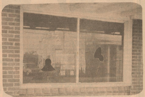
BROKEN WINDOWS -- Two windows were broken at Everet Calk's business sometime Friday and more destruction was reported at Pete's Texaco Service Station during the week end. Rocks were found inside Calk's building. At the service station a piece of concrete was thrown through the glass on the Coke machine, small windows were broken at the rear of the business and tires were scattered into the drive. Some signs were also reported to have been damaged.
