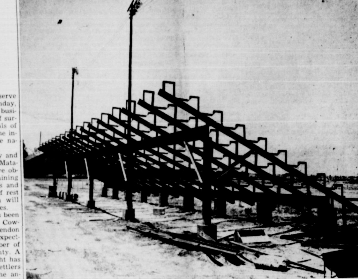
HOLD THAT LINE, MATADORS! Sounds like this will soon be originating from the vicinity of the steel framework shown in the above photograph. It is the new grandstand being erected on Burleson Field and is expected to be completed within a short time after wood for the seats arrive. The grandstand is being constructed by Field and Gym Supply of Vernon (formerly of Turkey) and was built in the firm's shop at Turkey and welded together on the site here. Johnny Truelove, manager of the firm said a minimum of time will be required to complete the grandstand after the remainder of the material arrives. Mr. Truelove is in California this week completing negotiations for the West Coast distribution of his invention, a device for the training of football players to block properly. The machine, which is equipped with hydraulic control, is finding immediate acceptance among coaches everywhere.—Photo by Douglas Meador.
