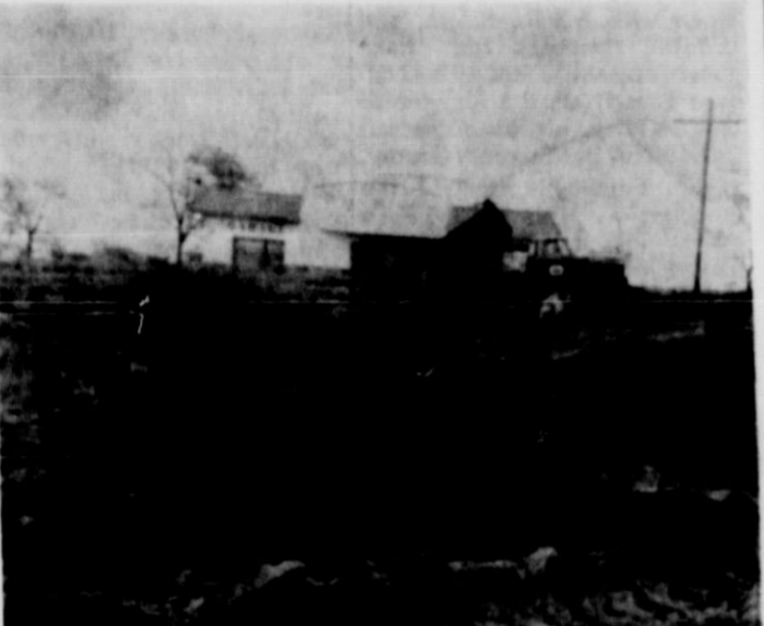
PRIME MOVERS —This photo was made north of the Tribune building yesterday afternoon, and shows a dump truck filling in the unsightly area along the bank of Ballard Creek, as a part of the most extensive terrain improvement in the city's history. The work extends the length of the creek through town and when completed is going to change the appearance of the entire area. Commissioner Clyde Gilbert and City Council member Freddie Welling, who is also President of the Matador Lions Club, are working jointly in the improvement.
