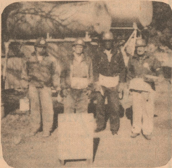
GREEN THUMB PROJECT --Members of the Green Thumbs were in Matador this week repairing the County Barn. Workers shown are (from left to right), Jim McCleskey, Rufus Melton, Toreman Lee Harris, and Dee Hall.
