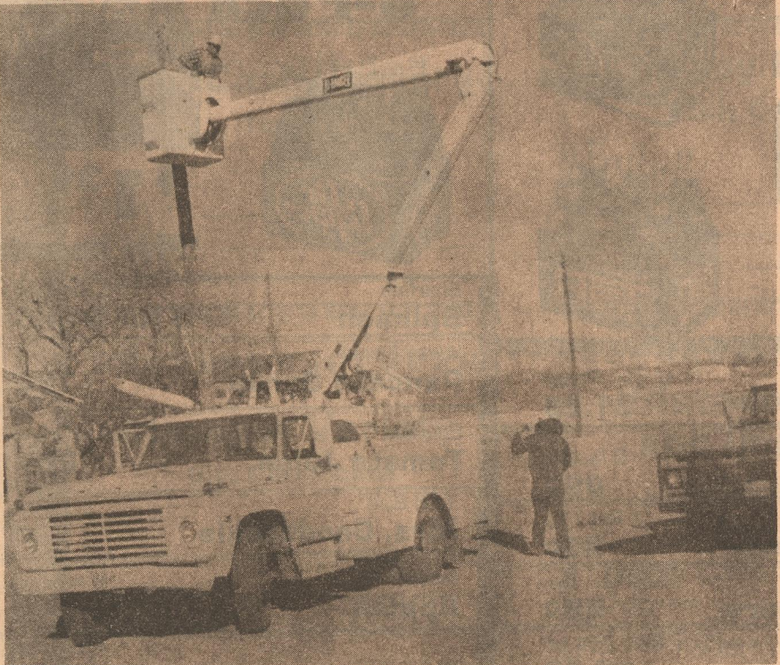
HIGHER VOLTAGE -- Electrical crews from P and B Construction in Childress spent more than a week in Matador changing downtown voltage lines from 23 to more than 70 to accommodate the new housing to be built northeast of the Motley County Courthouse. The new apartments are scheduled to be built in 1980, and will house average income residents. On the crew were the boss John Stedman, Butch Titsworth, Gene Richardson, Calvin Saunders, John Cunningham and Clyde Kain.
