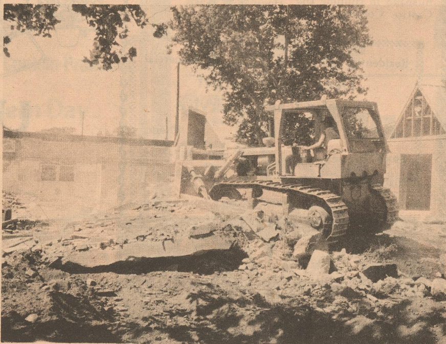
LAST REMAINS - The foundation and basement of the old Methodist Church in Matador were pushed down Monday. Beside the old building stands the new church which will be dedicated soon. The roof of the old building caved in last year, ending its long existence as a house of the Lord. (Staff Photo by Leon Watson)
