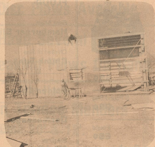
NEW BUILDING -- This new shop building is being built on Jess Couch's property north east of the courthouse near where new apartment buildings are to be constructed within four to six months. (Photo by Leon Watson)
