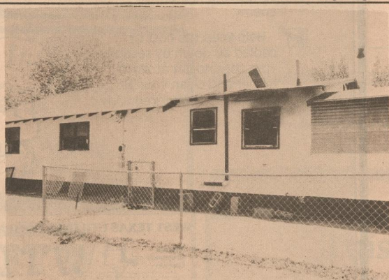
FIRE DESTROYS HOME: The Ewing home was destroyed by fire Saturday morning June 2. According to the Matador Fire Department the fire started in the vicinity of the hot water heater in the rear of the house. The back two rooms were near gutted and the rest of the house was damaged by smoke and heat. Carolyn Ewing was helping her daughter, Donna Ewing, move from Spur to Perryton, so she was not at home. Clay and Joely Ewing and Brad Wilson were at home. They all escaped the fire safely. The Ewing household items were not insured. The house belongs to Mrs. Wilma Hobbs. A love fund has been established at the First State Bank of Matador for the Ewing family.
