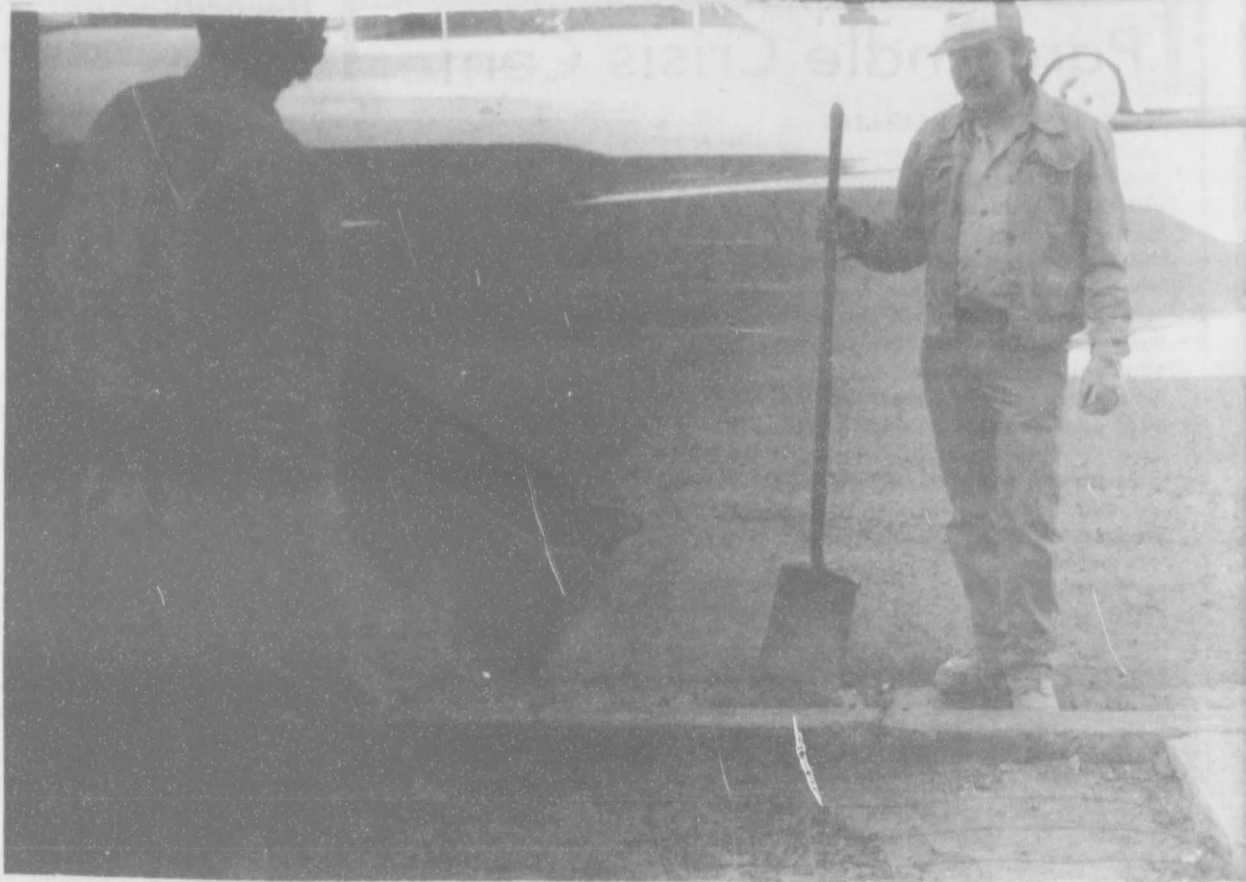
These construction workers were enjoying the good weather last Friday morning as they poured concrete for part of the new sidewalk in front of the elementary building.
