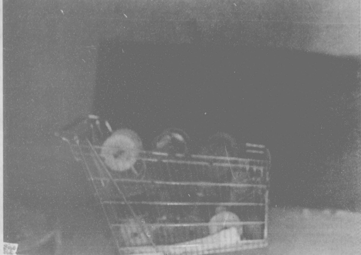
These are the chalkboards that are being installed in the new classrooms and a cart full of electrical supplies to be used in the new elementary school addition.
