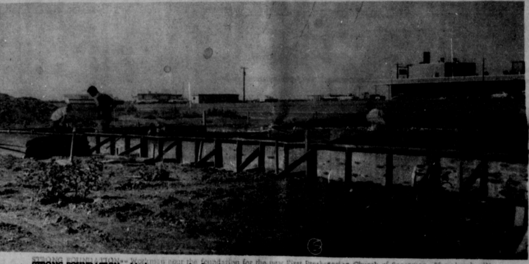
STRONG FOUNDATION-- Workers pour the foundation for the new First Presbyterian Church of Spearman. The church will be on Cotter Drive in the Blodgett & Linn Addition. The brick building will have a sanctuary, six classrooms, a kitchen, a nursery and pastor's office. PLAINSMAN PHOTO
