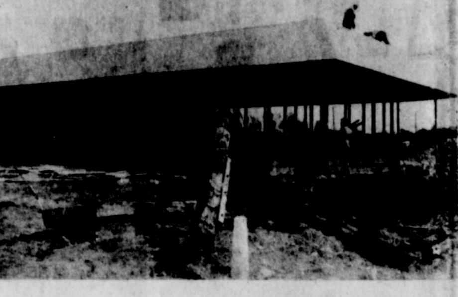
The walls were raised on the Dairy Queen this week. Completion date for the new business is tentatively set for January 1. (Staff Photo)
