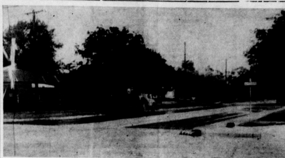
McLean's city street crew have been busy the last few weeks. They are shown here working on a section of 15 blocks that they are recoating.
