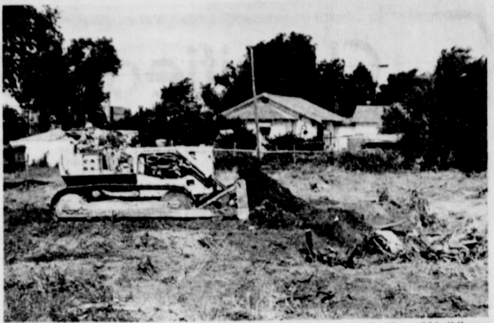
The city of McLean has been busy lately cleaning up vacant lots and tearing down old buildings. In the above picture, the old swimming pool on Kingsley Street is being filled in. (Staff Photo by Lisa Patman)
