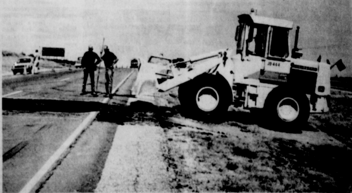
THE HIGH TEMPERATURES in McLean have been dealing the state highway maintenance crews misery. Here, men repair a section of I-40 east of McLean which exploded because of the heat. (Photo by Linda Haynes)
