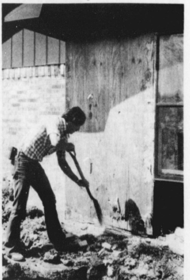
BILLY THOMAS, ADMINISTRATOR of Thomas Nursing Home, begins repairing the damage done to the Home when a bulldozer pulled a gas pipe loose and caused the bricks on this wall to fall. [Photo by Linda Haynes]
