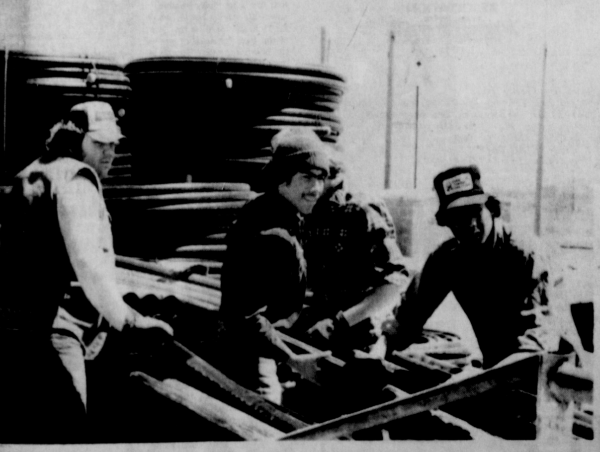
WORKERS WITH WES-TEX Construction unload more plastic pipe to install in the city's new gas line. (Photo by Linda Haynes)
