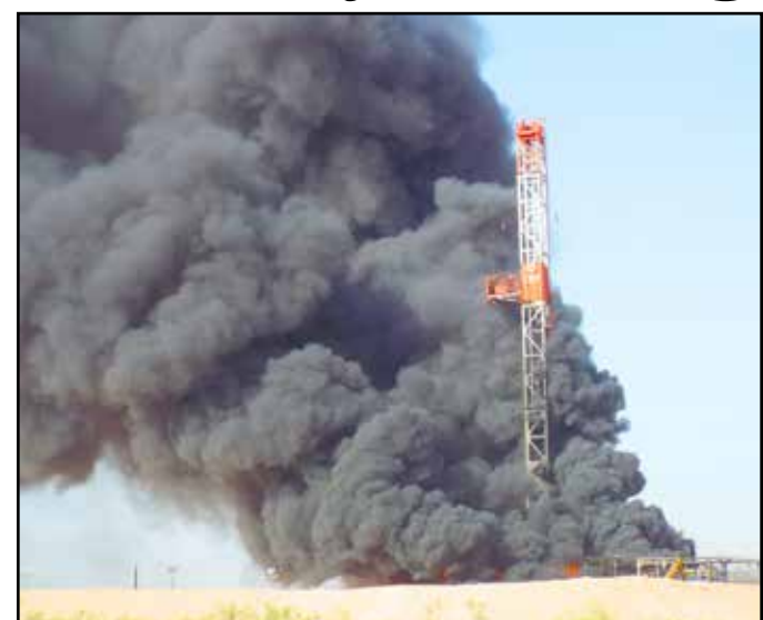
HERALD photos/Roger Cline Fire engulfed an oil rig in Northern Howard County, near the intersection of County Rd. 50 and County Rd. 19 this morning. Howard County volunteer firefighters battled the blaze. No information on injuries was available by press time.
