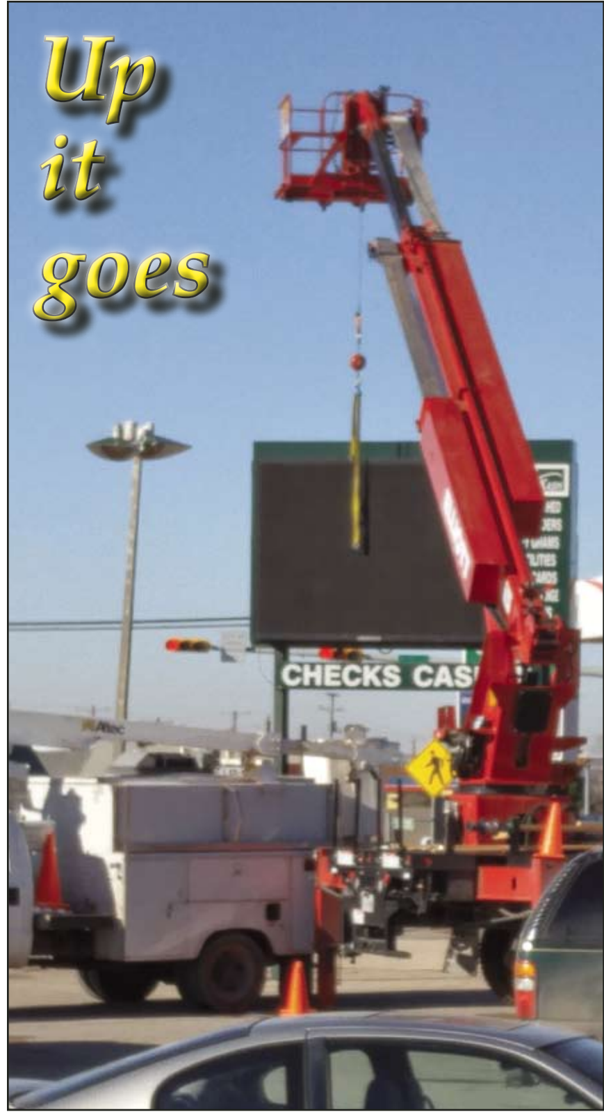
Up it goes HERALD photo/Steve Reagan This crew was busy Wednesday afternoon installing a new sign-board at Kwik Kash on South Gregg Street.
